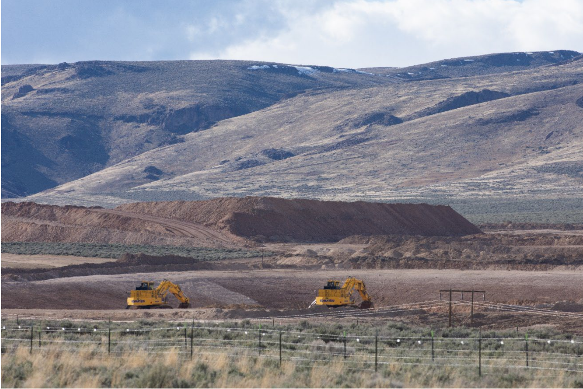
Construction for the mine at Thacker Pass in Nevada, March 2024. © 2024 David Calvert
