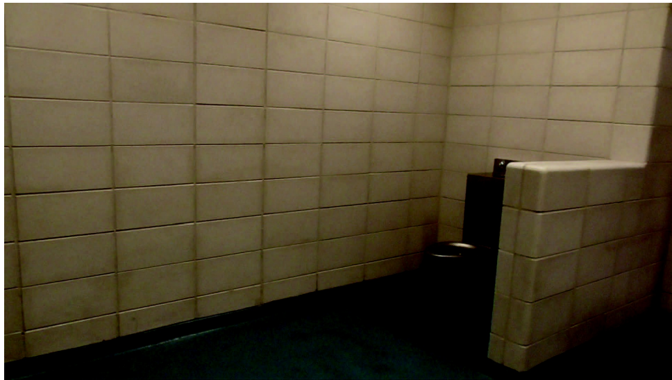
Toilet and sink behind half wall in tenth-floor hold room. PX301, at P000350.
