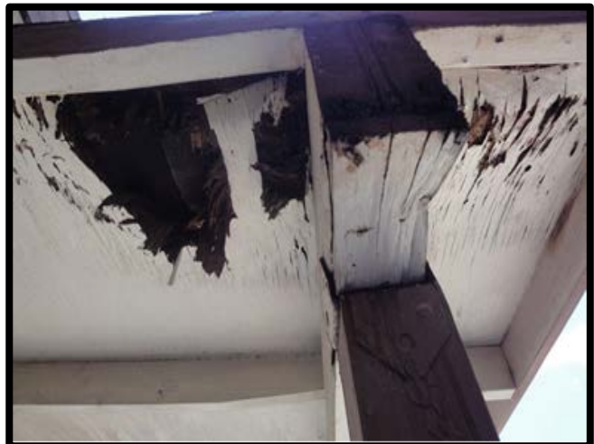
Rotting Structural Beams at the Kingsville, TX Maintenance Facility
