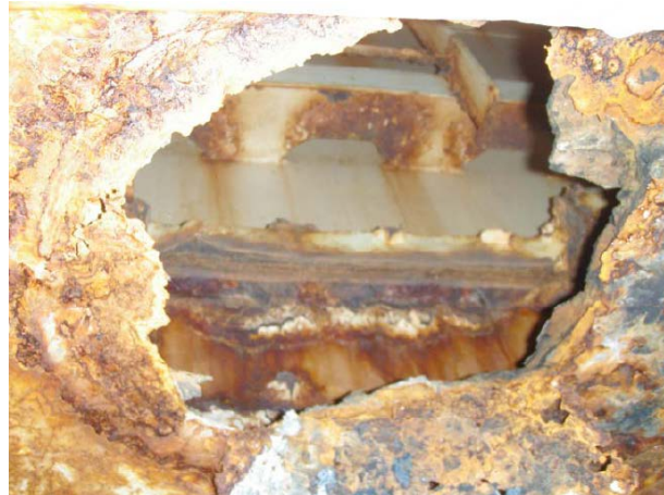
Wing-wall corrosion below safety deck
