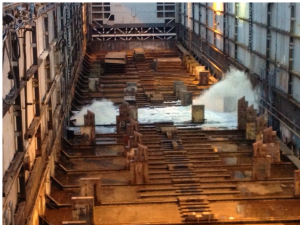
Testing ballast/flooding systems
