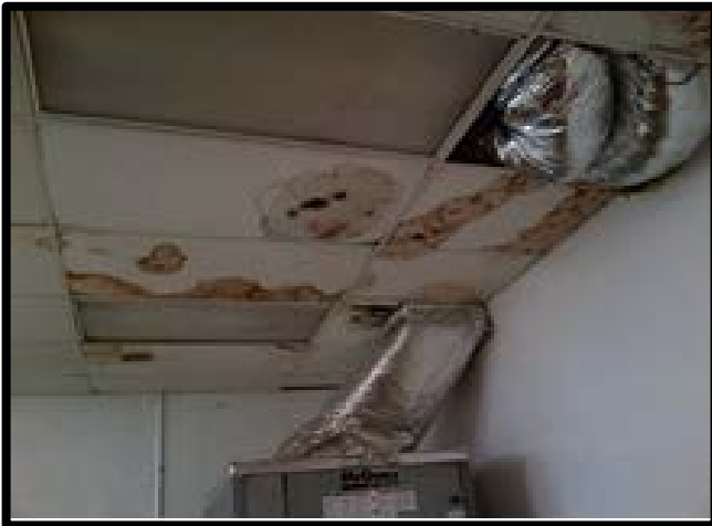
Mold and Leaking HVAC in the Administrative Office Building at the Aguadilla, PR Airport
