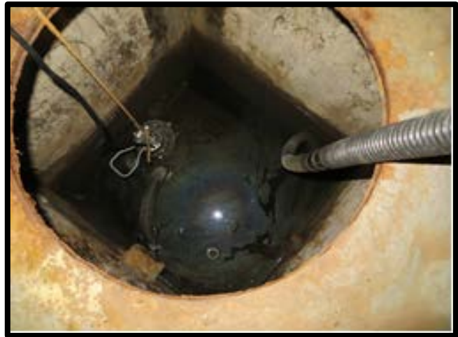
Broken Sump Pump and Drain System at the Ft. Covington, NY LPOE
