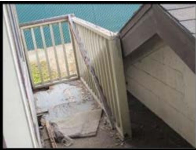
Balcony with structural damage at the Chula Vista, CA Border Patrol Station
