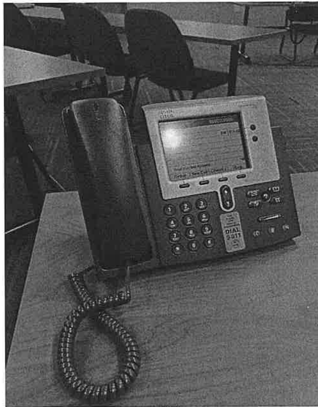
16 PHONES LOCATED ON TABLES OF THE EMERGENCY OPERATIONS CENTER
