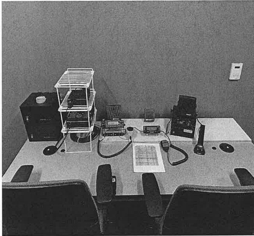
EOC COMMUNICATIONS ROOM
