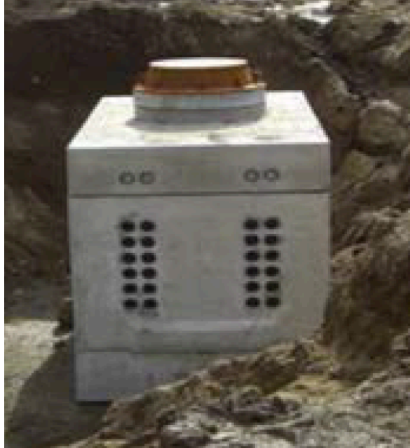
Figure 31 — Manhole for fiber patching in Virginia Beach 50
