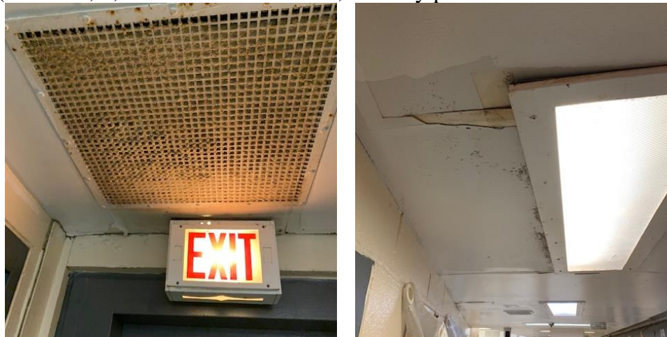
(Photo 35, Moldy and dusty air vent; Photo 39, water-damaged light fixture)
