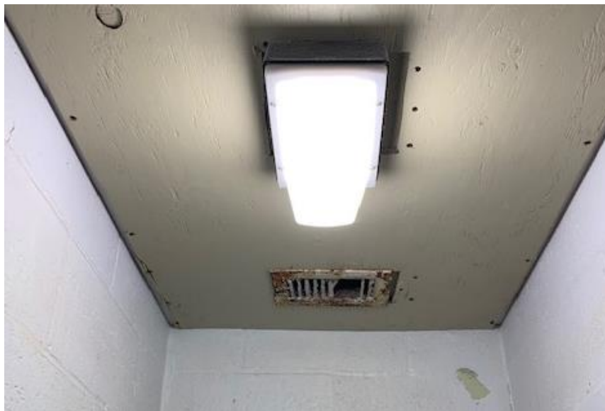
(Photograph 158, Room 309's bathroom ceiling)
