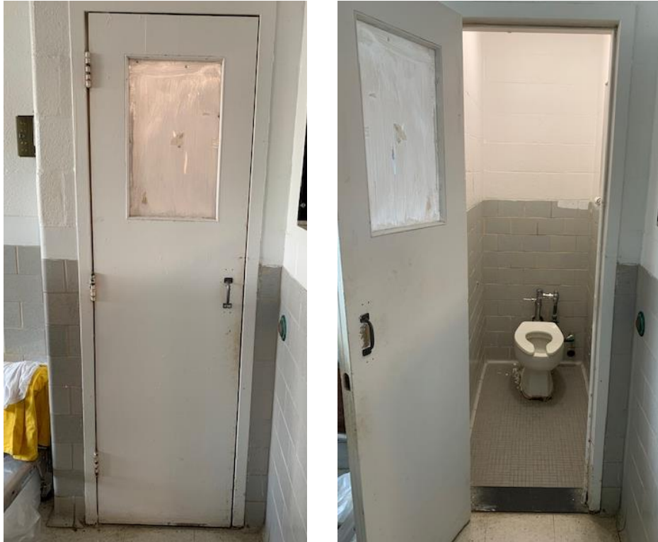
(Photographs 114-115: Room 407 Bathroom – Not ADA Accessible)
