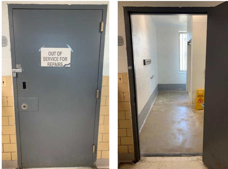
(Photograph 160: Out of Order 3rd floor ADA bathroom; Photograph 161: grab bar on left below towel rack)
