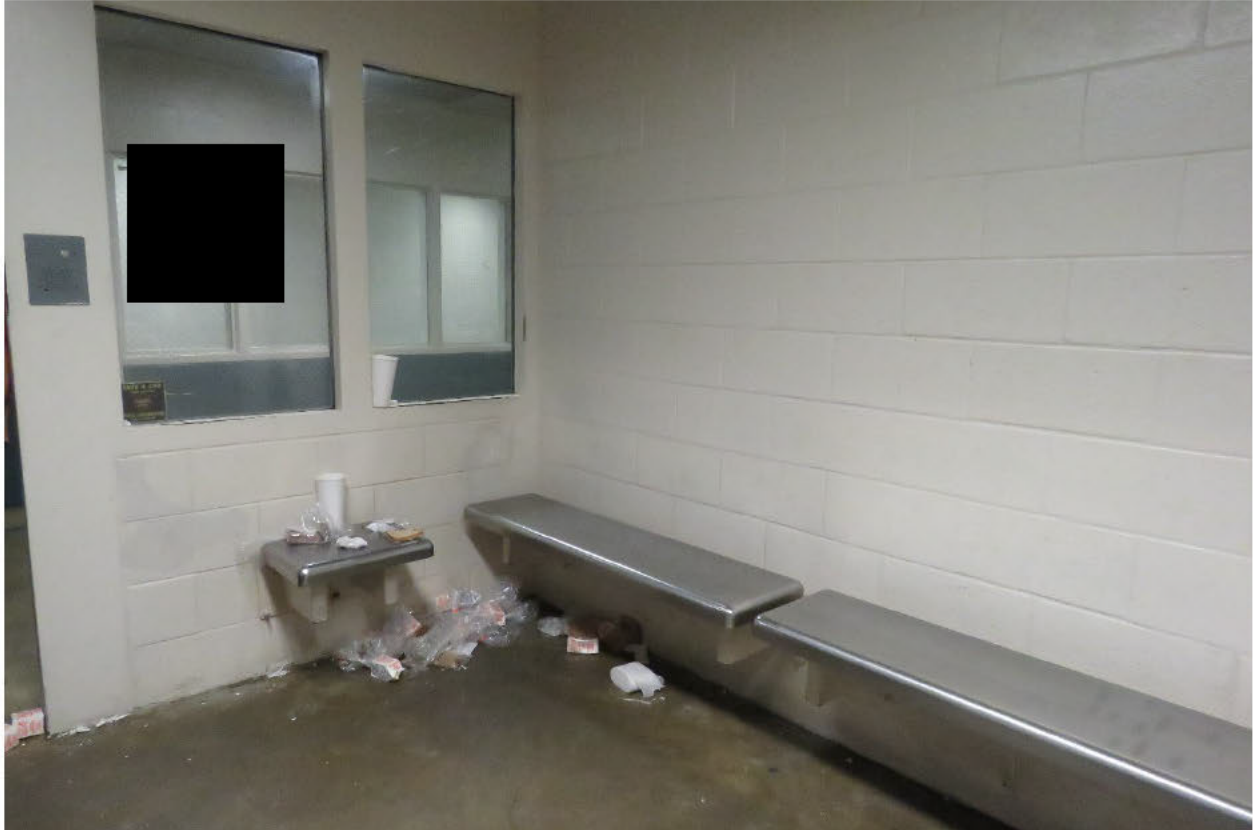
Photograph 14 – Cell 111, view from rear, more trash
