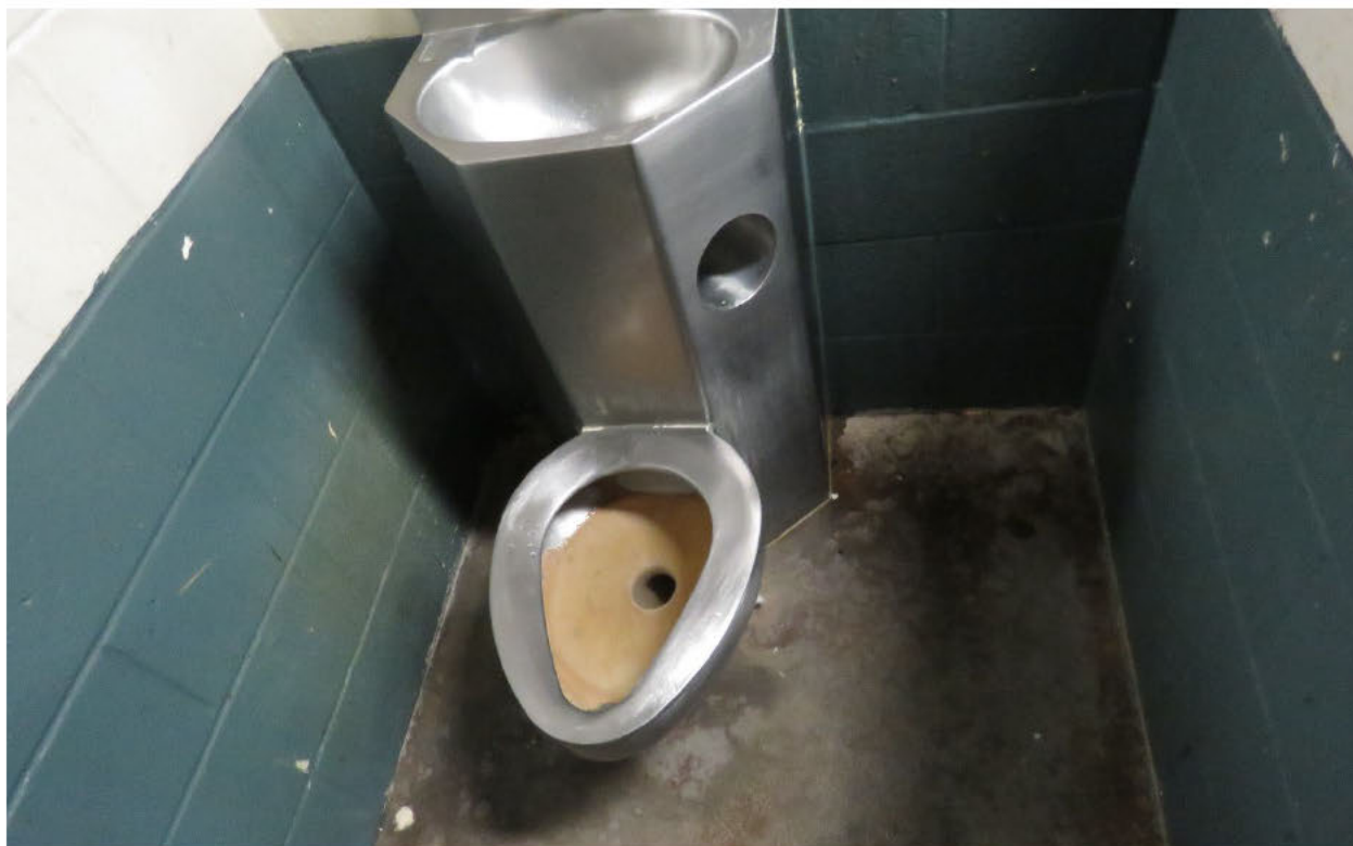
Photograph 2 – Same toilet at rear of main IRC Clinic area, looking into the bowl
