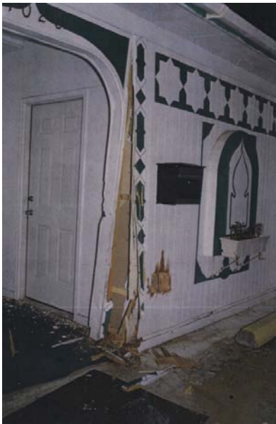
This Florida mosque was damaged after Franklin crashed his truck into it.
